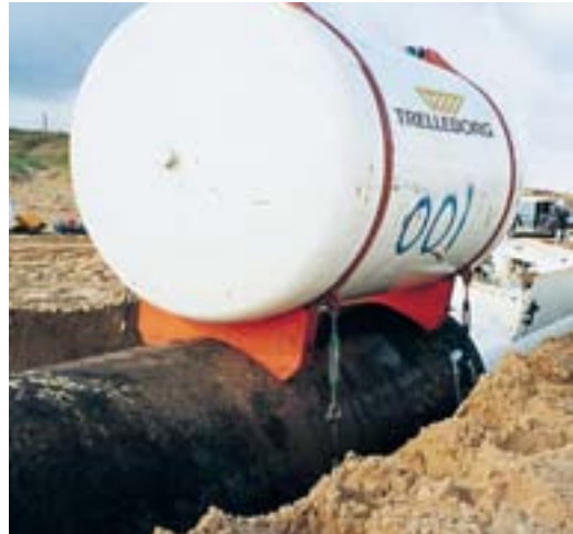
Pipeline Interface Saddles for Buoyancy Tanks
